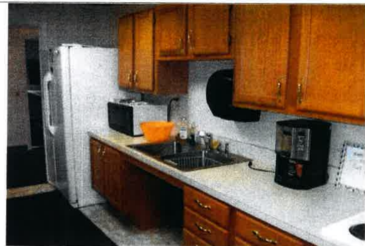
The handicap accessible kitchen was installed in 2007 and features 34-inch high countertops; a forward-facing, roll-under sink with covered piping; and side-by-side refrigerator; however one upper cabinet needs to be lowered.
