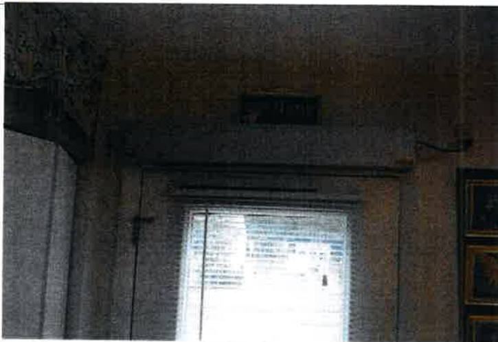
The one and two bedroom handicap accessible units (11-C and 14-F) both feature power-assist door openers at their front entrance doors.
