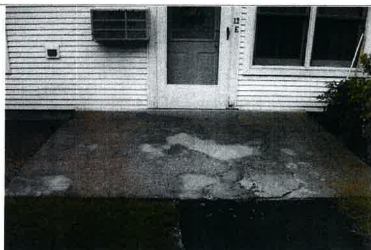
Similar premature concrete deterioration issues exist at the dwelling unit rear-elevation patios. These will need to be fully replaced as well.
