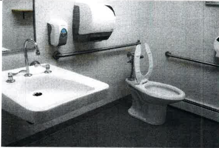
View of typical finishes and fixtures within the two fully-accessible restrooms. Note that the side grab bar is fixed too low and needs to be raised to the same height as the compliantly positioned rear grab bar.
