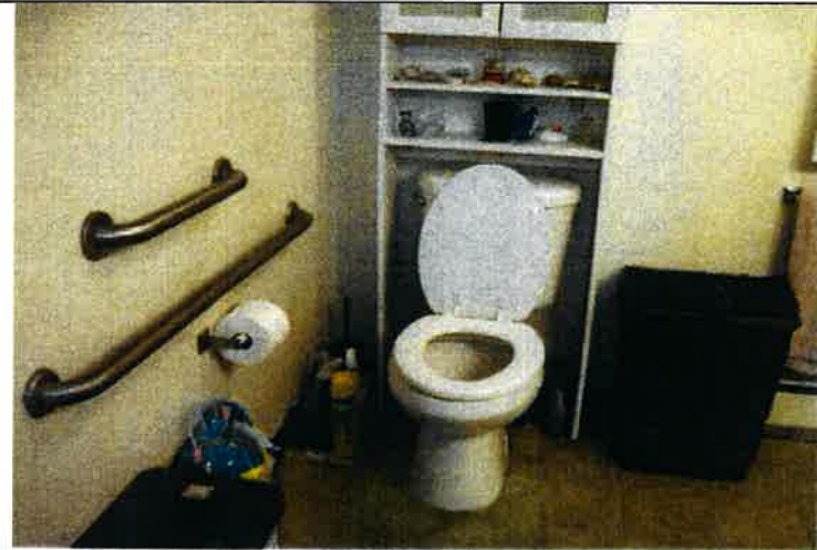
The bathroom in accessible one-bedroom Unit #11-C features vinyl sheet floors and toilet grab bars; however the existing side grab bars are incorrectly positioned; and there is no compliant rear grab bar.
