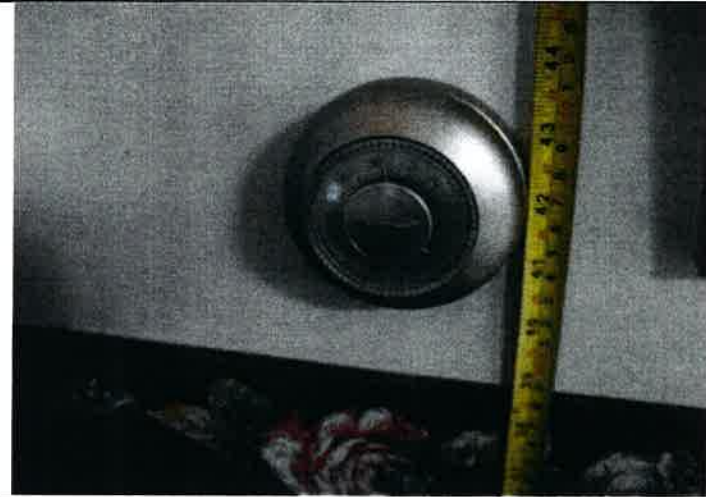
Dwelling units feature Honeywell dial-type thermostats. The accessible unit thermostats are positioned correctly; however they need to be replaced with compliant digital, push-button models that do not require grasping or twisting.
