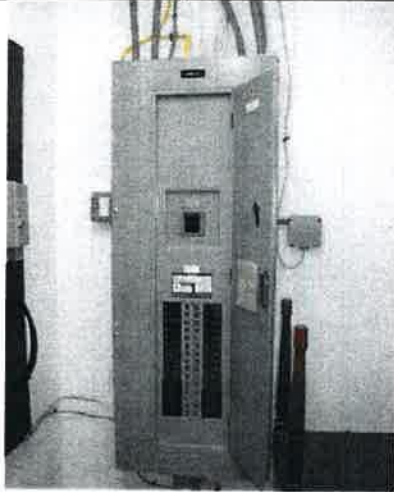
Each building features sheathed-cable copper wiring and Siemens circuit breaker and main disconnect equipment.
