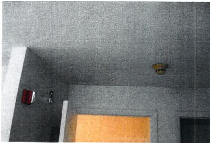
All dwelling units feature hardwired smoke detectors, heat detectors; and audio -visual horn/strobe warning devices connected to the central fire alarm control panel.
