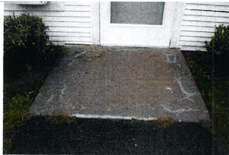
Several of the concrete pads at the dwelling unit front entrance doors have cracked and deteriorated beyond repair and will need to be fully removed and re-poured.
