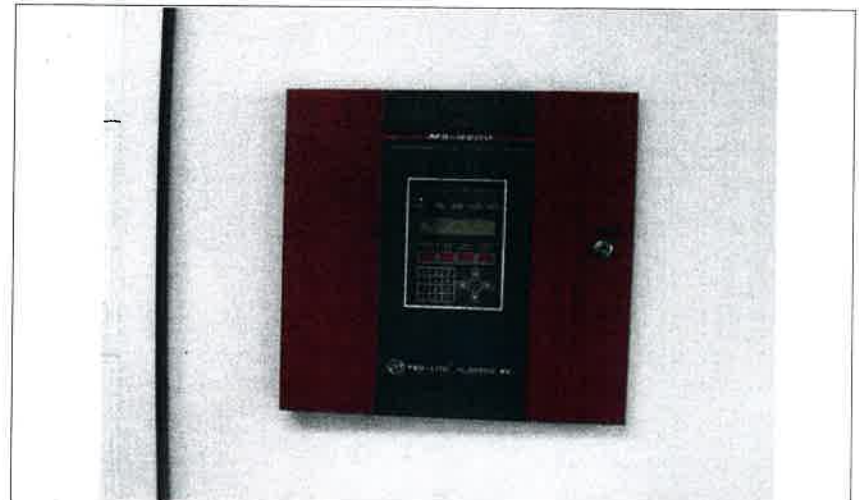
A single Fire-Lite MS9200 addressable fire alarm control panel monitors hardwired end-devices located in all six buildings. The panel reportedly dates to the 1995 construction and has far surpassed its 15-year useful service life.
