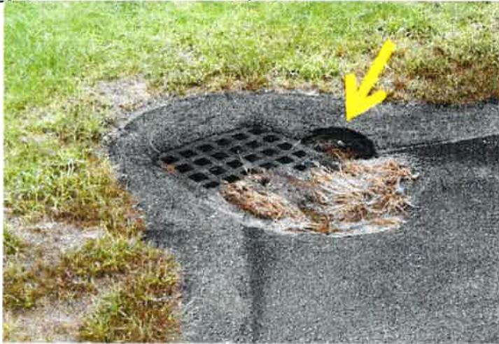
View of sectional asphalt subsidence observed at a drain grate located at the east end of the loop roadway. In need of near-term repair/possible re-setting.
