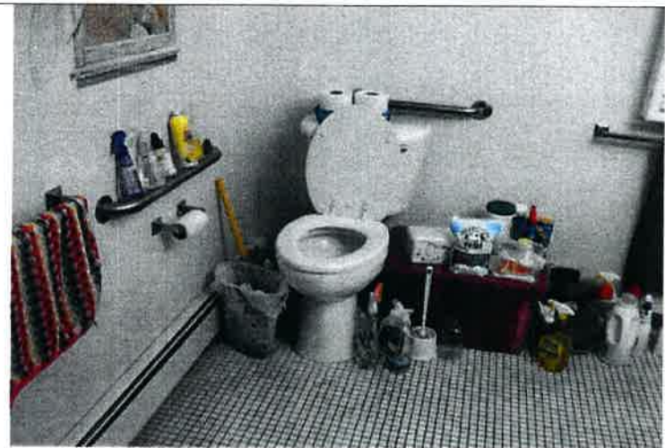
The bathroom in accessible two-bedroom Unit #14-F features ceramic tile flooring and front and rear toilet grab bars; however both bars are non-compliant in length and incorrectly positioned.
