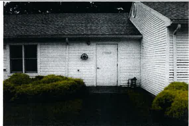
A central storage room with flush-metal door is located on the front side of each building. The gutters and downspouts at each building reportedly date to the 1995 construction and have surpassed their 20-year EUL.
