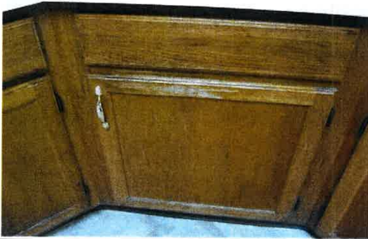
Age and use-related finish wear is visible on some kitchen woodwork. The cabinets all date to the original 1995 construction of the development and are now approaching the end of their 25-year expected useful life.
