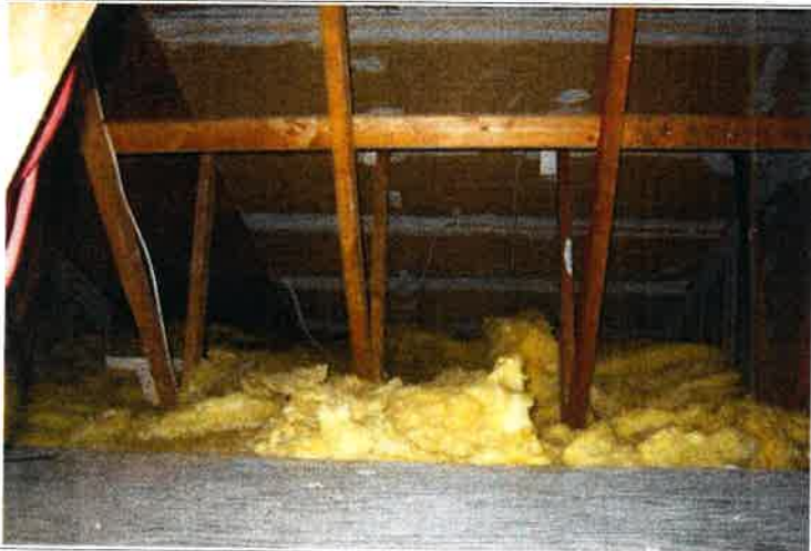
All buildings feature wood framing, plywood roof decking, and insulated attic spaces. All kitchen rangehoods and bathroom exhaust fans are ducted out through the building soffits and are covered with insulation.
